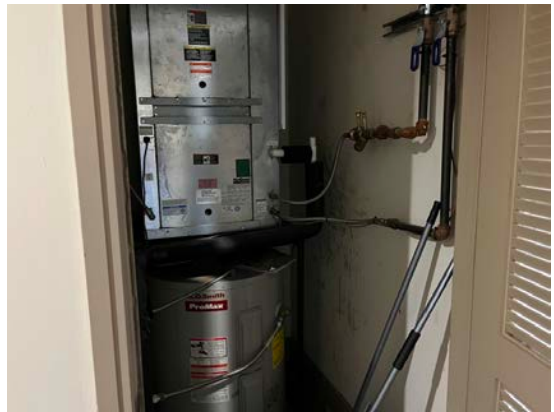
Unit 14003 HVAC Closet
