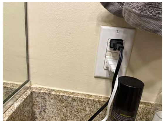
Unit 18002 GFCI - Bathroom Wet Area
