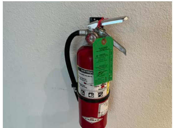
Common Area Fire Extinguisher
