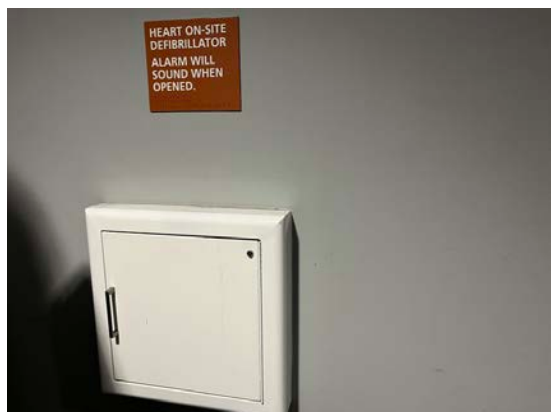
Floor AED Cabinet
