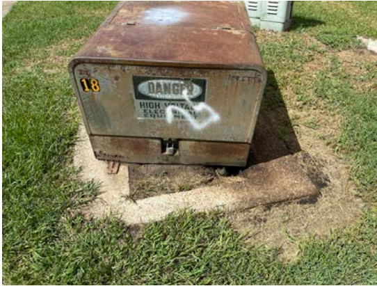
Apparent Leaking Transformer
