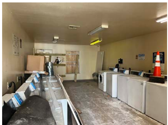
Community Laundry Facility Interior
