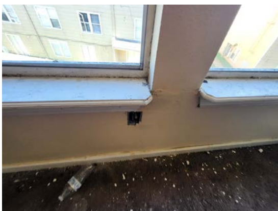
Caulking (Suspect ACM)
