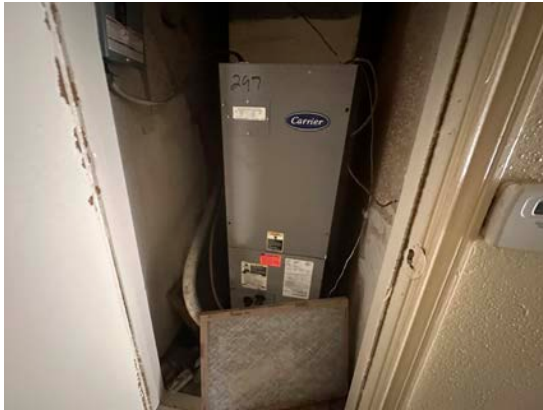
Unit Air Handler
