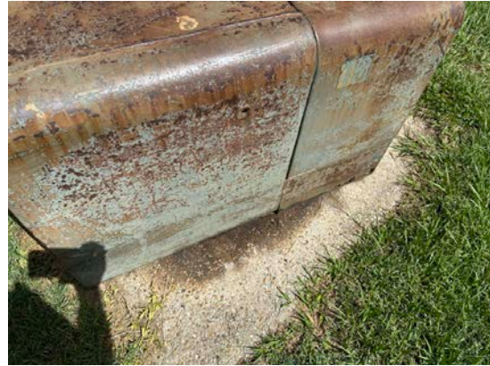
Apparent Leaking Transformer
