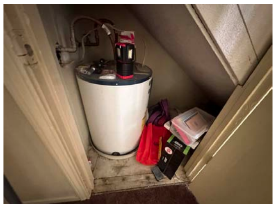
Unit Water Heater
